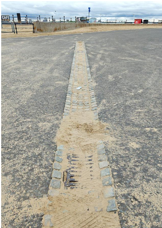
Photograph 6: Sand blocked gully drain at the north end of Perch Rock car park.
