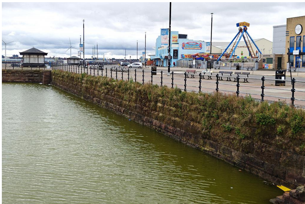
Photograph 13: Weed growth along the southern blockwork wall.
