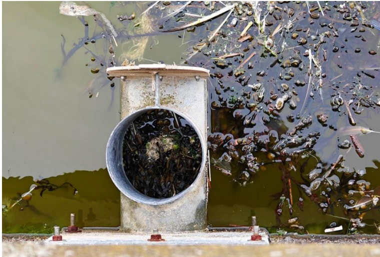
Photograph 7: Open flap valve on inflow pipe on northern wall of lake.
