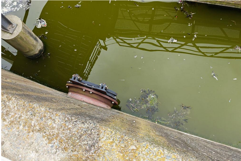
Photograph 5: One of two drainage inflow pipes located at the western end of the lake.
