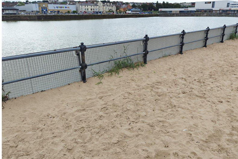
Photograph 3: Mesh railing panels installed to reduce windblown sand inputs into the lake
